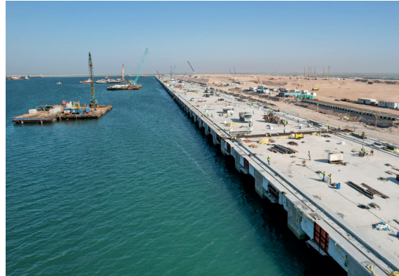
Construction Works Continue at the Grand Faw Port Project in Basra, Southern Iraq.
